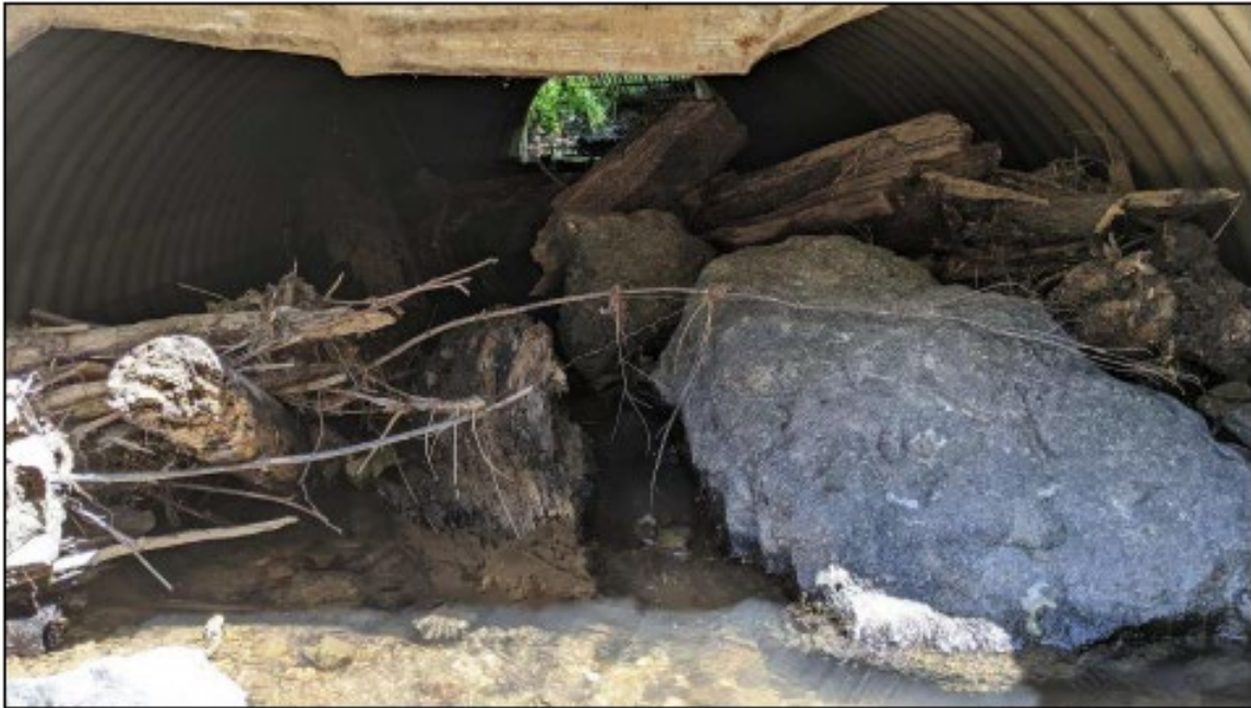
Photo 7: View looking upstream from the downstream side of the partially blocked culvert.
