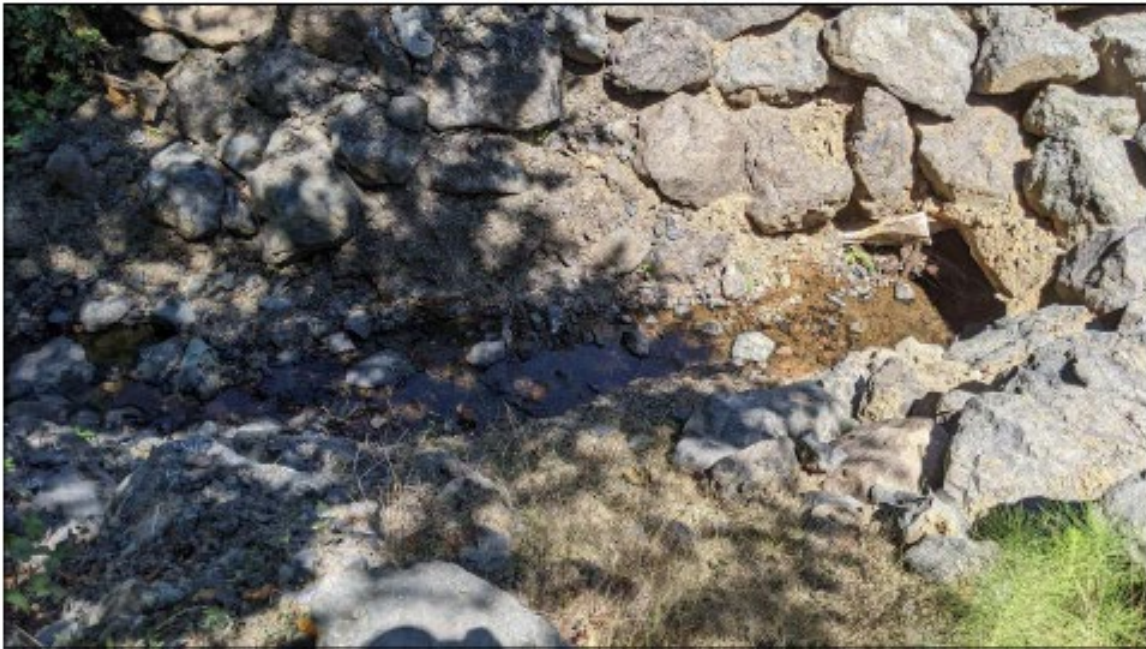
Photo 8: Stream conditions immediately downstream of the culvert. Large rock was used to stabilize roadway after culvert collapsed.
