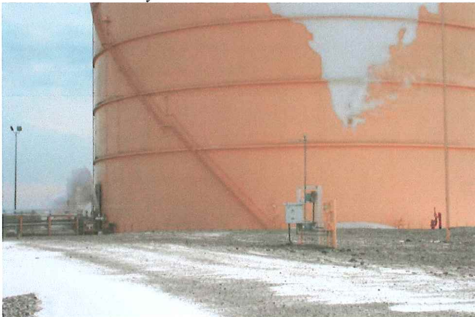
A V-shaped ice formation develops above the puncture on Plymouth LNG tank while pipe (lower left) spews LNG and gas vapor. By Washington Utilities and Transportation Commission (Used with permission.)
