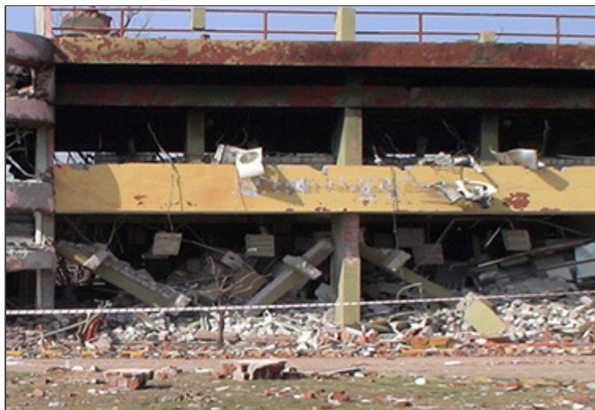
A 2009 vapor cloud explosion and ensuing fire at an Indian Oil Corp. facility in Jaipur, India, destroyed the plant and damaged homes more than a mile away, according to an investigation report. Photo courtesy of the U.K. Health and Safety Laboratory.
