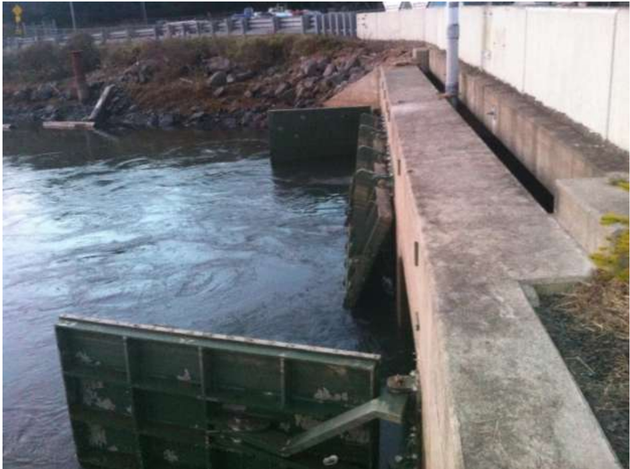
Figure 1. Existing tidegates (4) at the East Bay Road bridge over the Kentuck Slough channel. The tidegates and bridge were rebuilt in 2007 at the cost of over $2 million. (1-8-15).
