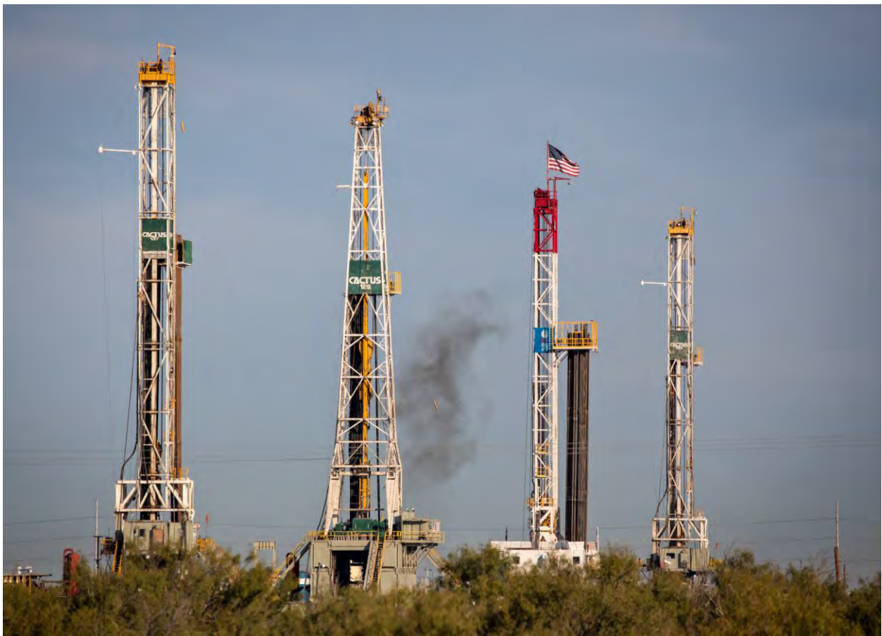
Fracking rigs off of Interstate 20 West of Midland, Texas, in the Permian Basin ©2018 Julie Dermansky
