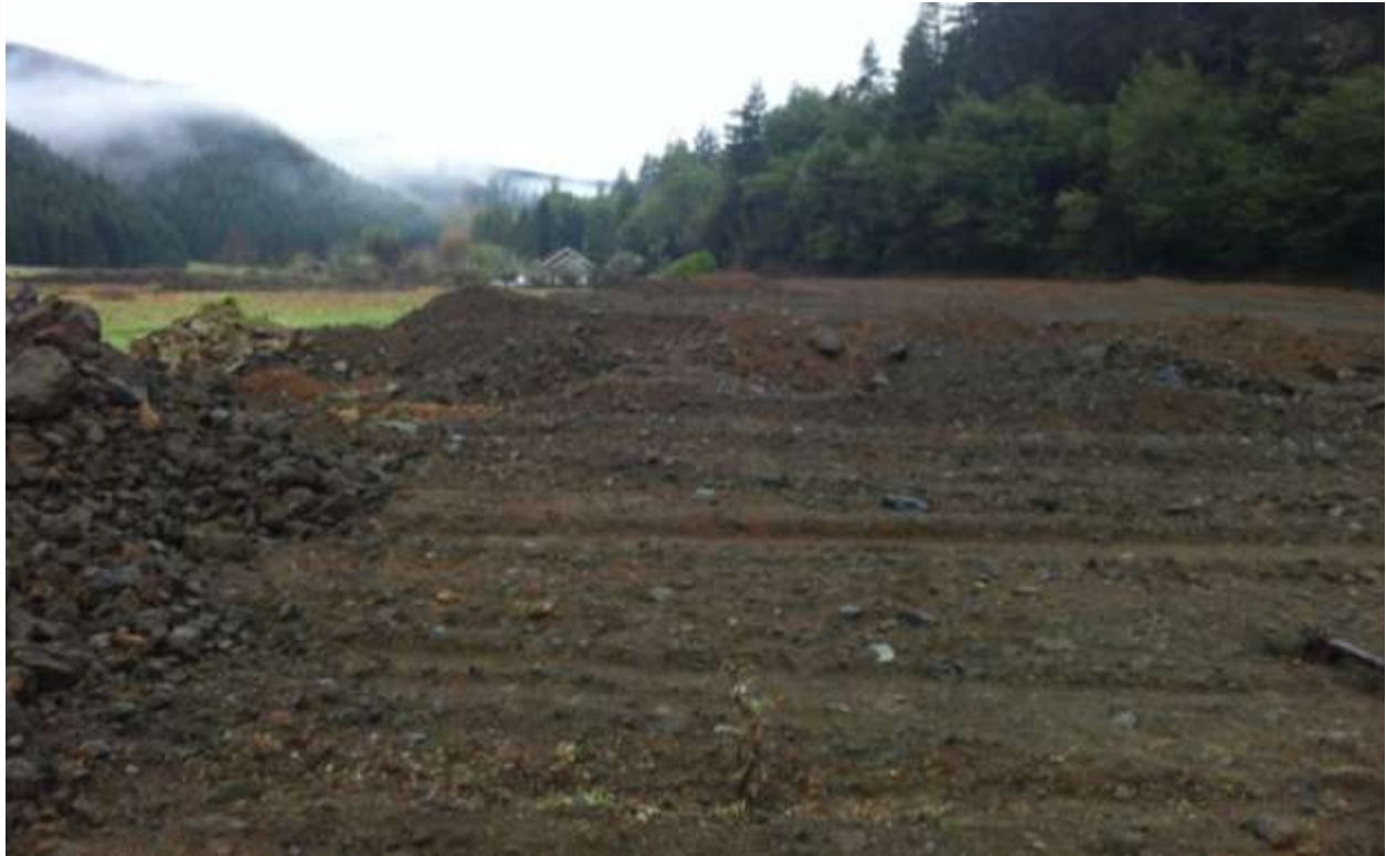
Figure 9. Ongoing fill activities along Kentuck Way Lane. View is at MP 3.2 looking west. (1-11-15)
