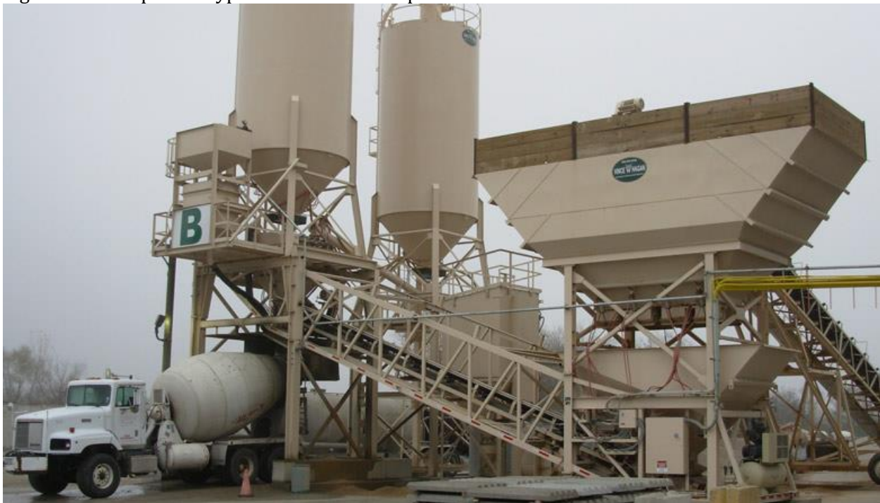
Figure 1 - Example of a typical concrete batch plant
