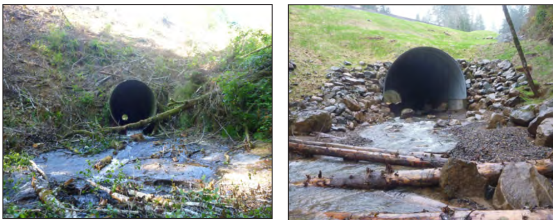
Figure 17. Undersized culvert with step blocked movement of Coho and Chinook to high quality upstream habitat (left). Culvert was removed and replaced with 26' wide arched steel set onto concrete footings (right), allowing natural stream habitat to be maintained through the 126' long passage. Source: CoosWA 2013
