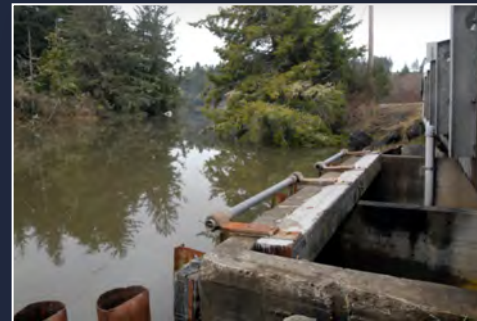
Tide gate regulates tidal flooding at Willanch Slough.
